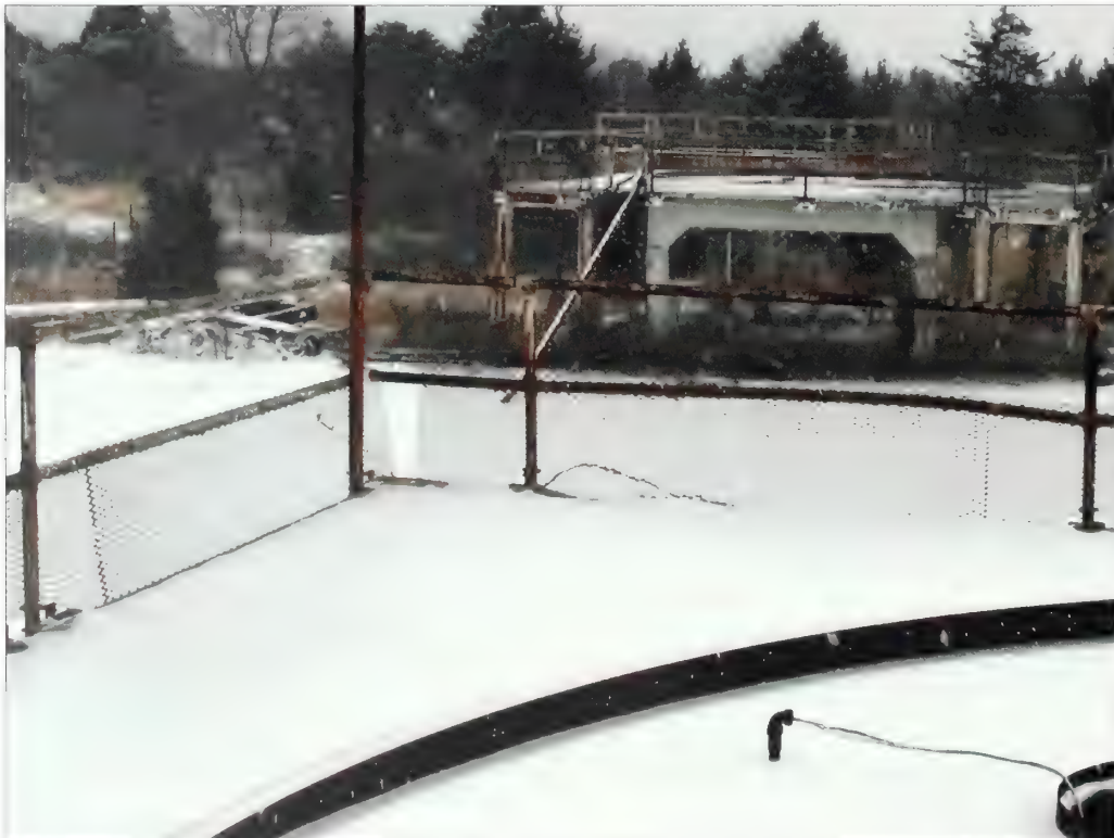
Figure 5.107. Existing expanded metal mesh on guardrails at radar tower, NIKE radar site. New expanded metal mesh should match the existing in this photograph and be applied to the lower and upper openings of the existing guardrails for added safety (Olmsted Center, January 2009).
